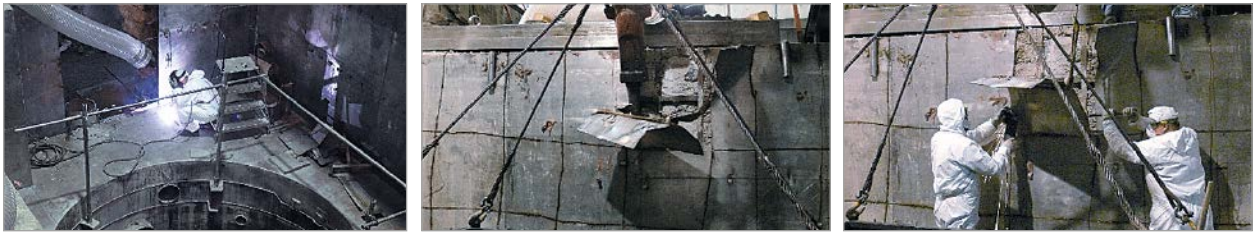
Figure 8. Dismantlement of MR reactor lining: using a plasma cutter and RCM BROKK equipped with a hydraulic hammer
