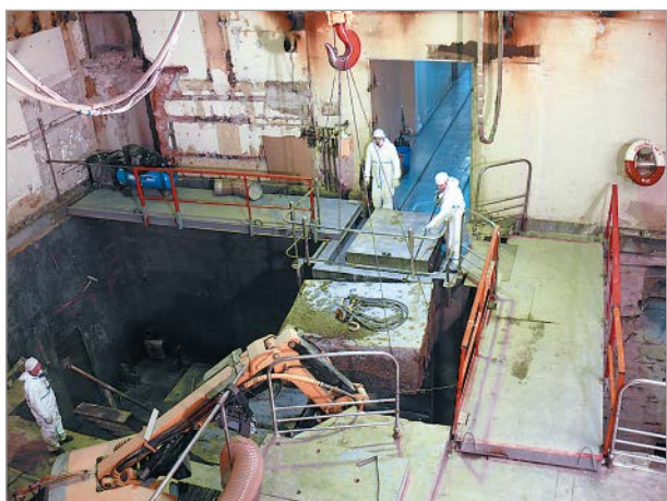
Figure 12. Dismantlement of MR reactor's concrete shielding using a wire rope cutting tool
