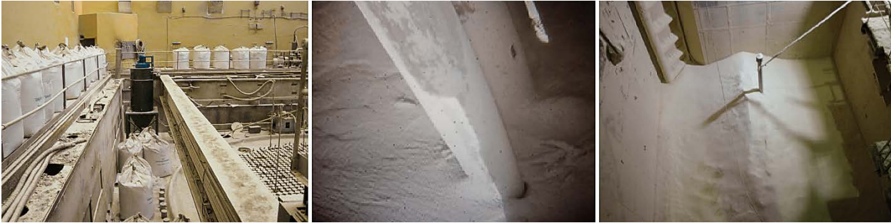
Figure 3. Construction of additional safety barriers inside PUGR EI-2 pit: the main hall during the backfilling process (left), barrier material inside the void spaces of the reactor pit (center), inspection channel inside the technological shaft (right)
