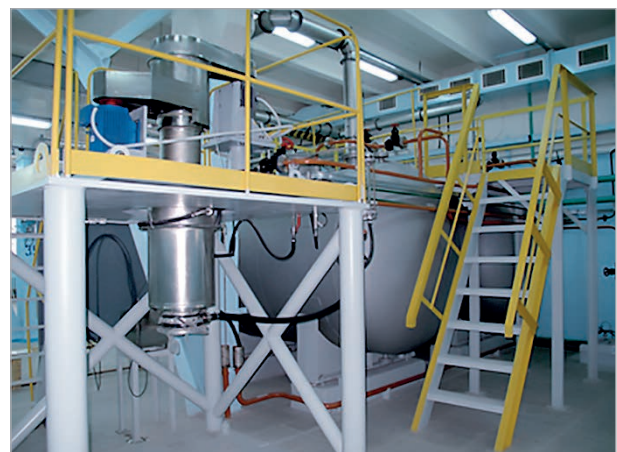
Figure 3. Pulp segregation facility
