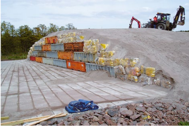
Figure 1. VLLW disposal technology at the DFRW site (Oskarhamn NPP, Sweden): installation of the covering screen [2]
